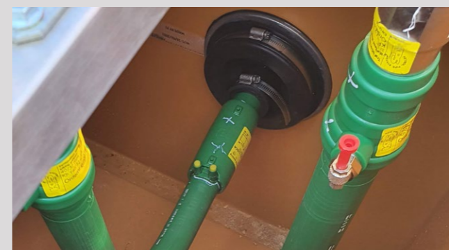
Public refuelling installation
