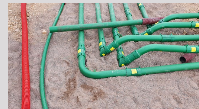
Public refuelling installation
