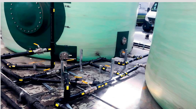
Maxol AdBlue Manufacturing Facility, Ireland
